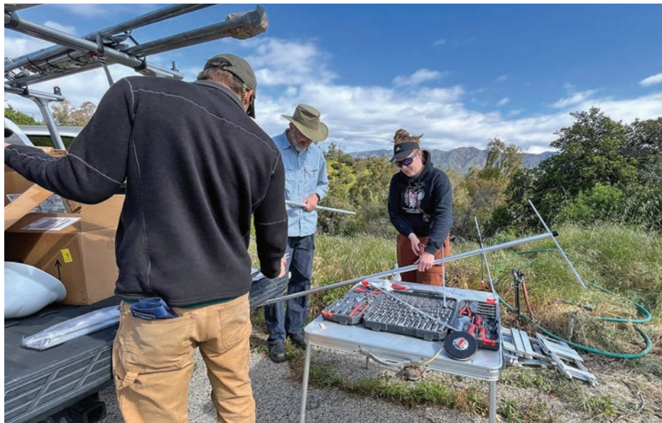
A team installs L.A.’s first Motus tower on Zoo grounds. Now active, this station will capture signals transmitted from animals in Griffith Park and beyond. Photo by Earyn McGee
